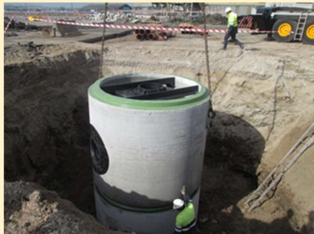
Actual hydrodynamic separator at dock installation
